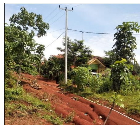
Figure 7. On-site System for Clean Water Distribution System at Housing Relocation Site, 2019.
