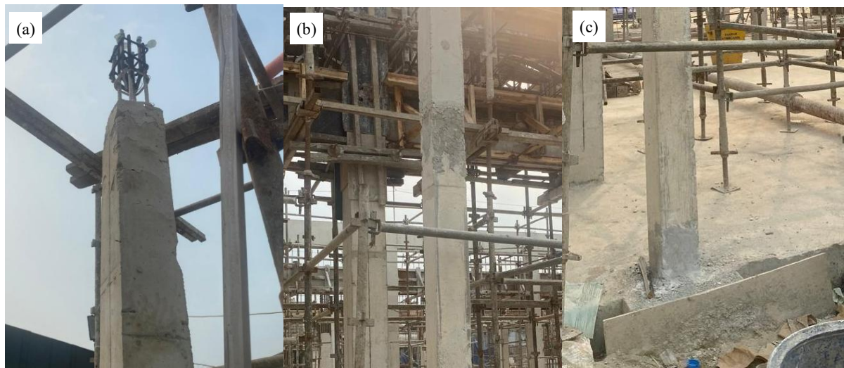
Figure 4. Representative Workmanship-Related Deficiencies Identified During Visual Inspection: (a) Severe honeycombing and inadequate concrete consolidation; (b) Construction joint with localized segregation and surface defects; and (c) Severe segregation at the column base with evidence of improper patch repair
